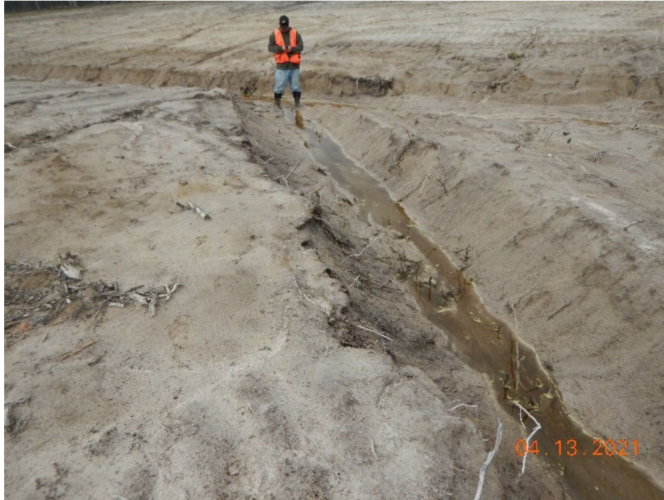
Photograph 1: EPA 2021 inspection photo (DSCN2686) taken on April 13, 2021, showing constructed drainage ditches in Wetland A.
