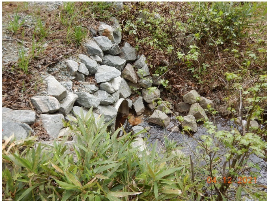
Photograph 4: EPA 2021 inspection photo (DSCN2573) taken on April 12, 2021, showing outlet of culvert under Ashcake Road flowing from the Site; looking southwest.
