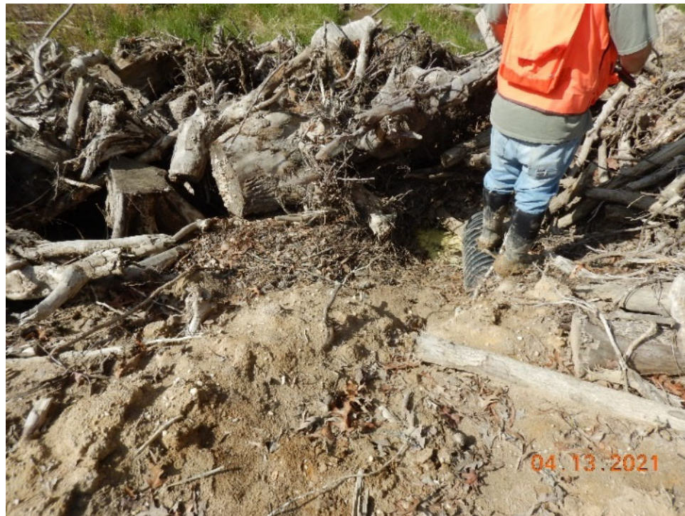
Photograph 2: EPA 2021 inspection photo (DSCN2746) taken on April 13, 2021, showing a constructed berm across Wetland A with a single pipe in the berm (below the inspector's foot) directing and altering flow/hydrology.
